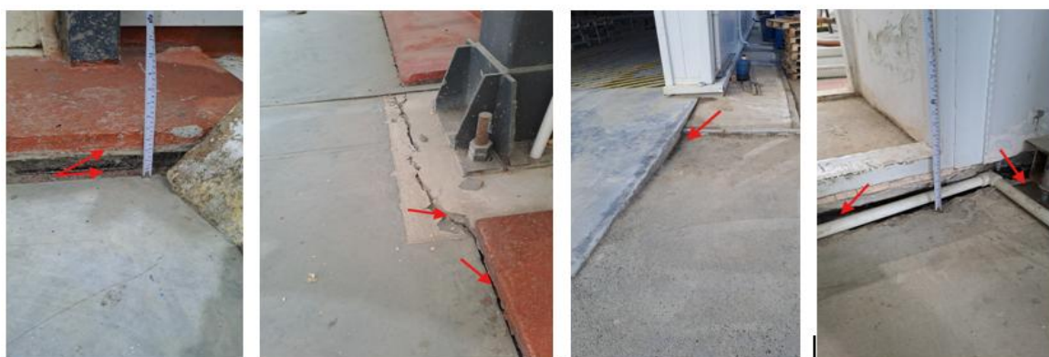
Figure 2 Foundation deformation Source. Authors.
