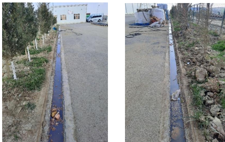
Figure 4 Localized water ponding
